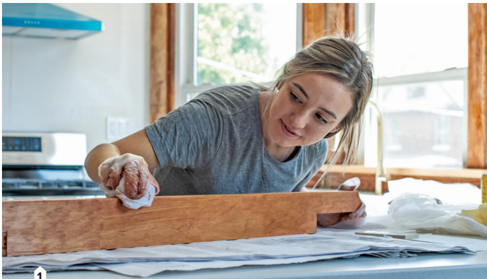
1 | Gruenwald stains wood in the upstairs dining room. To the relief of her many TikTok followers who value historic preservation, she went with a light, subtle stain to match the existing trim.
